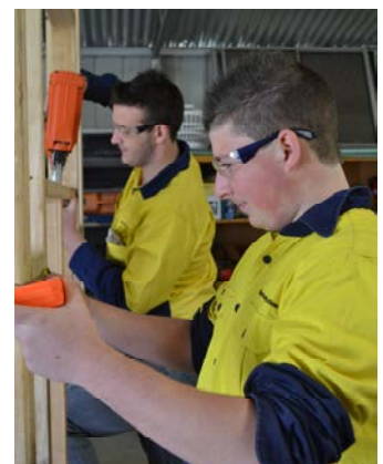
Right: Certificate I in Construction (Doorways 2 Construction) students building a wall frame at Henley High School.
